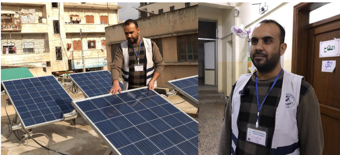
Nurse Tarek checks the solar panel system, ensuring it powers the center and helps maintain optimal conditions for vaccine storage.
